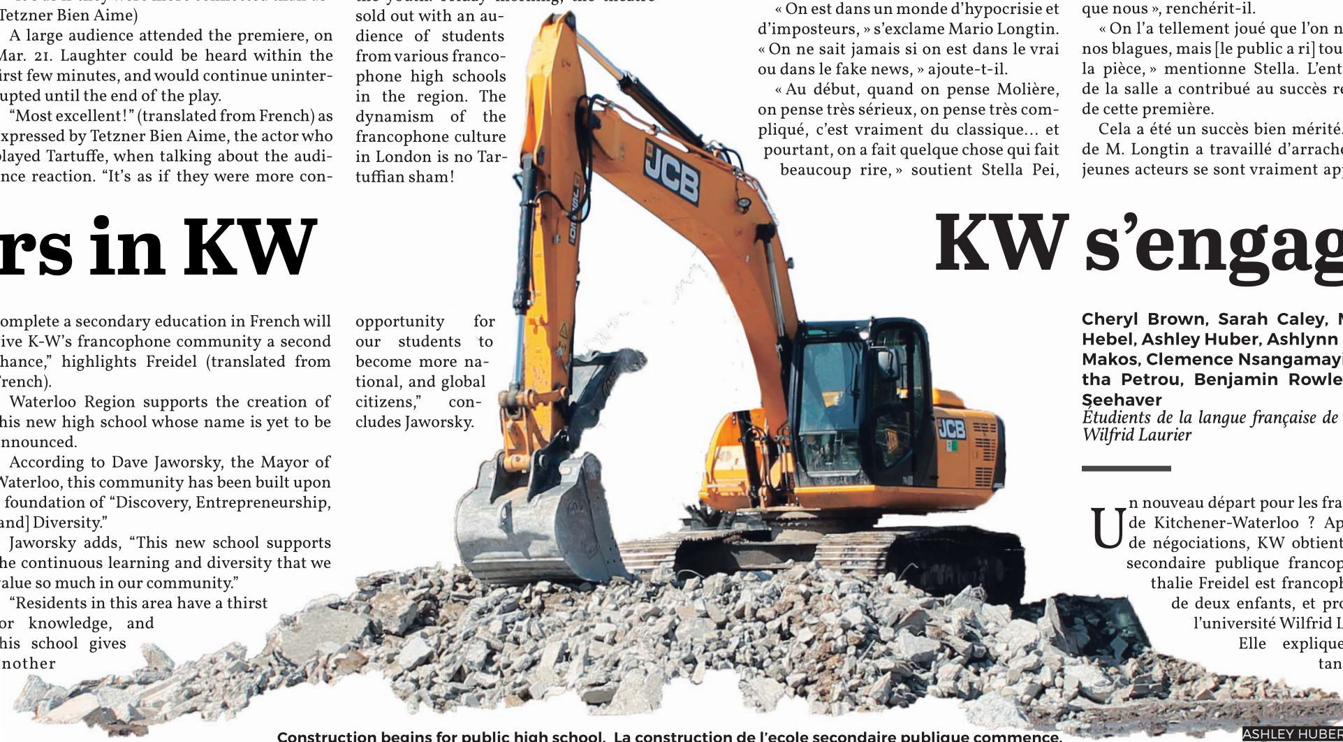
Construction begins for public high school. La construction de l'école secondaire publique commence.
